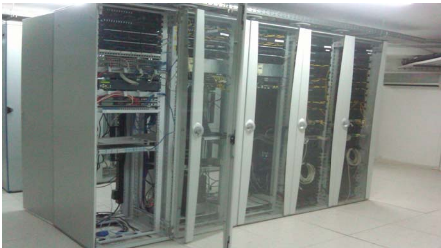
Figure II.4 - Fibre optic exchange located within the Industrial Consortium of Sulmona
